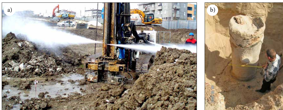
Fig. 1. Specificities of jet grouting technology: a – in the course of jet grouting, cement slurry is injected into soil through small-diameter nozzles (Jet grouting... 2016), b – cement slurry is mixed with soil, and cement treated grout columns are received
