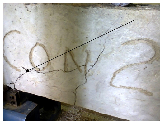
Fig. 8. Shear cracks in control beam (0% mix)
