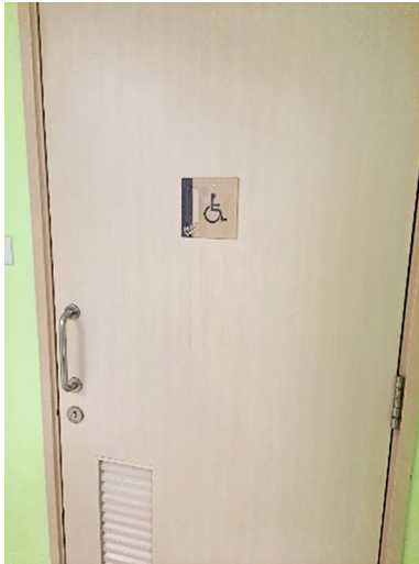
Figure 5. Example of “accessible” door in reality
