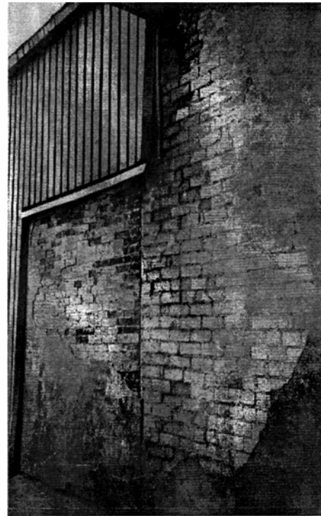
Fig 5. Destruction by exfoliation of usual plaster on ceramic and sand-lime brick masonry facade of the industrial building of institute Termoizoliacija in Linkmenų St 28 after 10 years of service
