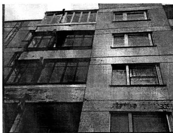
Fig 1. Destruction by exfoliation of decorative facing carpet of enameled ceramic tile of house facade in Ukmergės St 55 after 20 years of service under natural conditions
