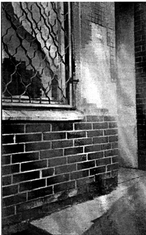
Fig 4. Destruction by exfoliation of polyclinic facade decorative facing out of carpet usual ceramic tiles in microarea Šeškinė after 10 years of service
