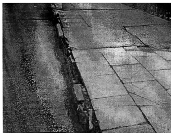
Fig 2. Destruction of reinforced borders of the bridge Valakampiai across the River Neris after 25 years of service
